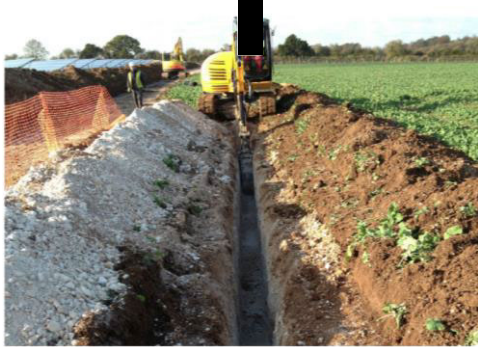
Cable trenching, showing topsoil stripped and set to one side, with subsoil placed on the other side ready for reinstatement (photo courtesy of British Solar Renewables)
