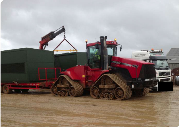
Case Steiger Quadtrac used to deliver inverters and other heavy equipment to site under soft ground conditions (photo courtesy of British Solar Renewables)
